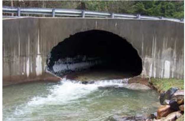
Perched culvert at Cummington Road (Riverways photo)
