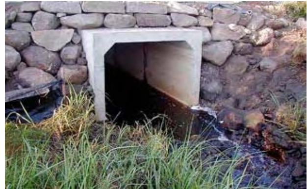
New box culvert that allows full tidal flushing (MA CZM photo)
