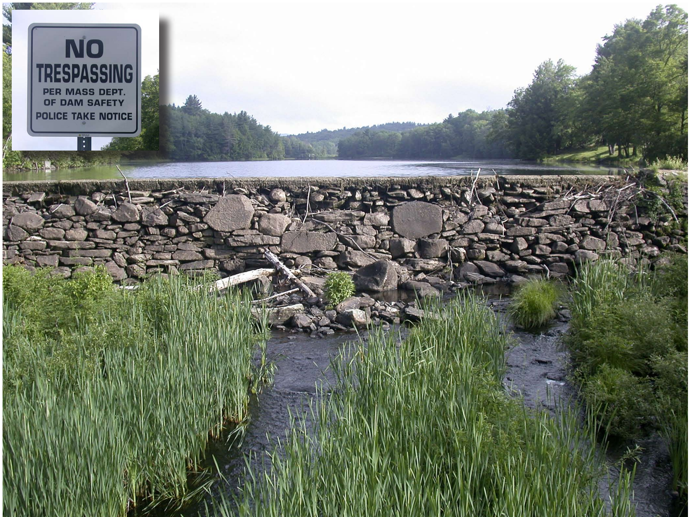
The old stone dam at the outlet of Hayden Pond in Otis, Massachusetts, is a decrepit structure that may fail. The Massachusetts Department of Dam Safety prohibits trespassers because of safety concerns. Its failure would likely have short-term yet catastrophic effects on downstream areas, and possibly threaten populations of the endangered brook floater.
